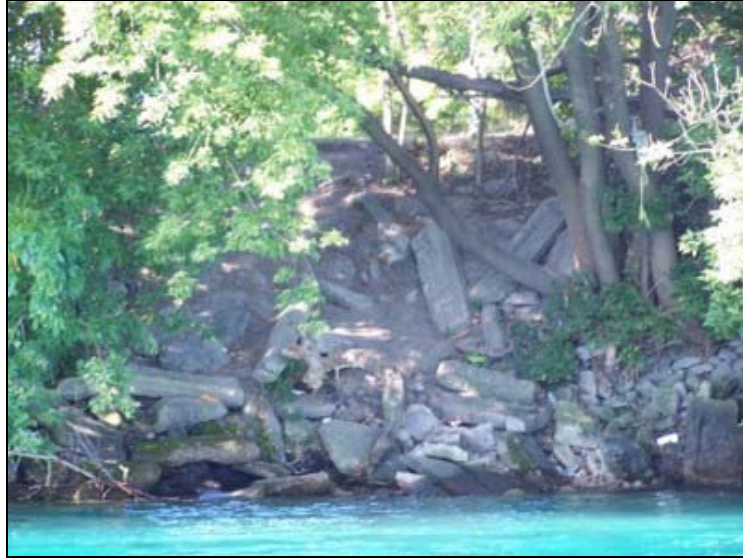
Figure 2.36 Eroded Area at “rope swing” South of Lincoln Street
