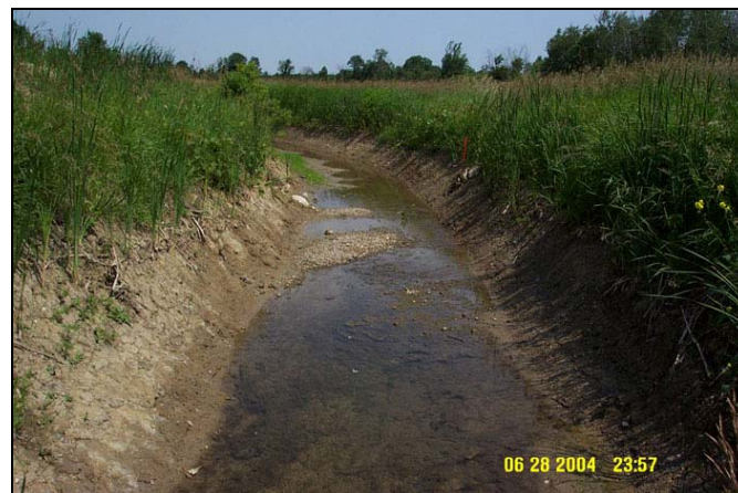
Figure 2.29 Example of Drain Maintenance along the Thomas Drain in the LHD Subwatershed
