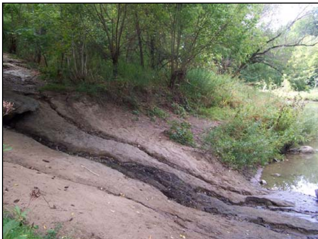
Figure 2.18 Erosion at Road/Stream Crossing at Norman Road in the LBR Subwatershed
