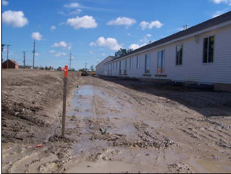
Figure 2.3 Urbanized Source of Nonpoint Source Pollution: Offsite Soil Erosion and Sedimentation at Construction Sites (photo taken of construction site at the corner of Bunce Avenue and Busha Highway in the SRD subwatershed)
