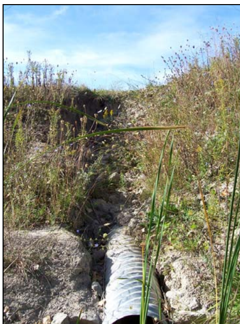
Figure 2.20 Erosion Around Drainage Structure
